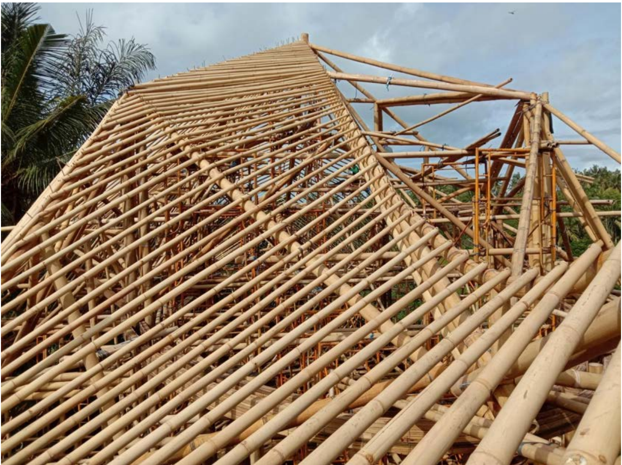
Bamboo tali poles for rafters during installation onsite. Tea House – Ubud, Bali. 2020.
