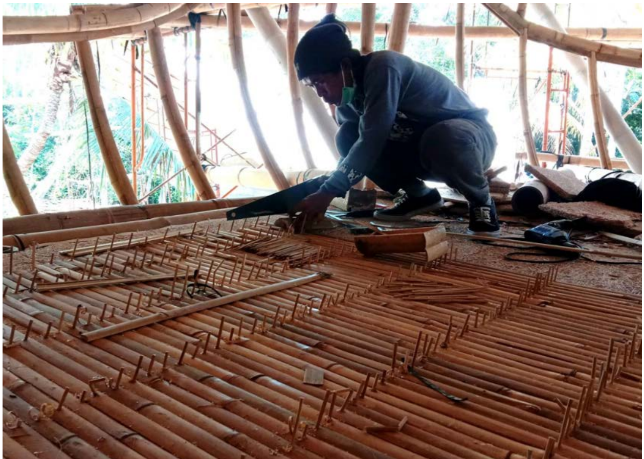
Bamboo pins Ø 4mm installation for bamboo flooring, Ulaman Eco Retreat, Kaba Kaba, Bali.
