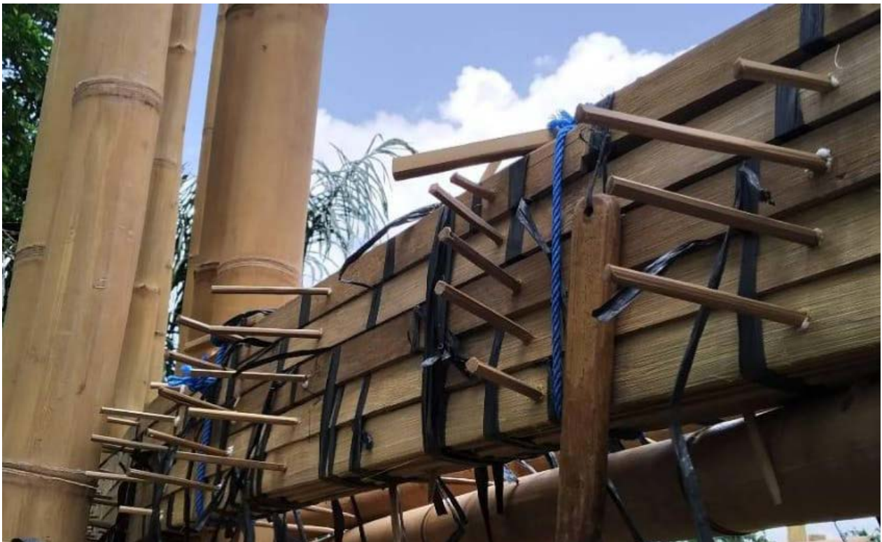
Bamboo pins Ø 8mm during installation onsite for split beam. Tea House – Ubud, Bali. 2020.
