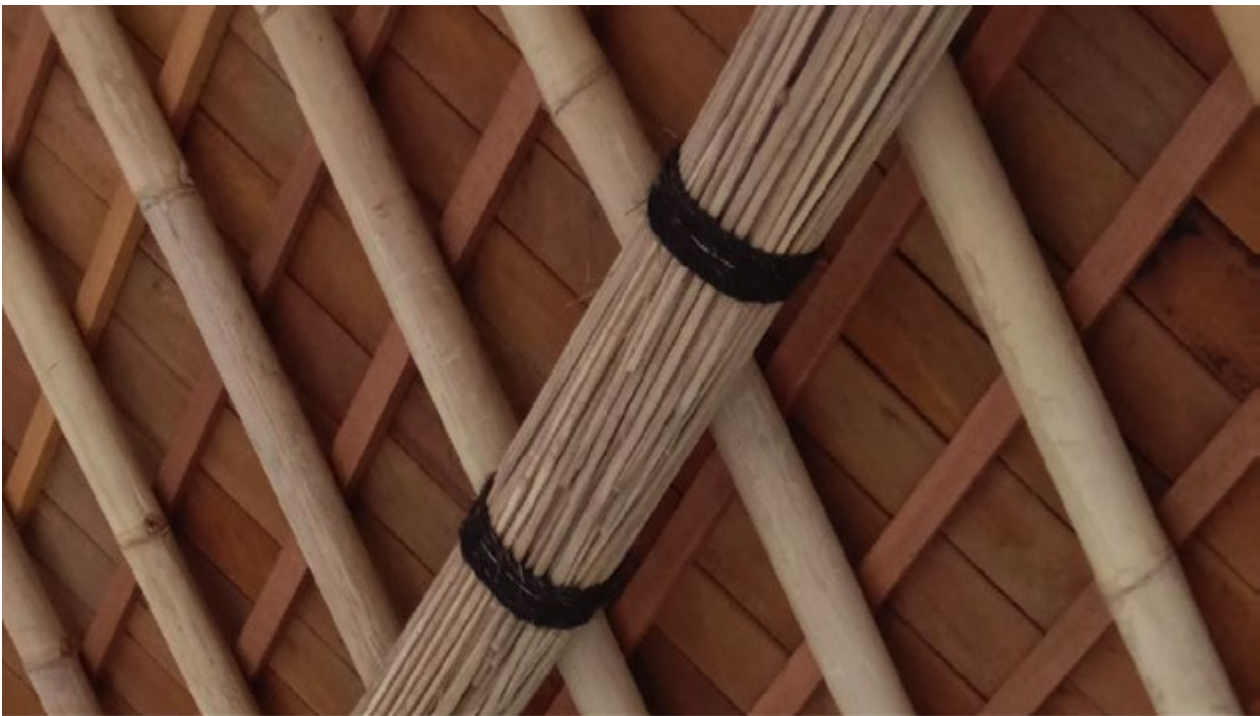
Bamboo lidi beam supporting the rafters and the roof. RASLI villa, Ubud, 2020.
