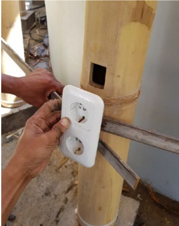
Electric installation sample.
